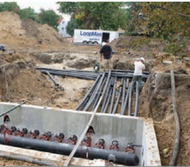
150 geothermal wells were installed under a parking lot to provide high efficiency heating and cooling using the earth's own renewable heat as an energy source. (UCM Photo Services.)
